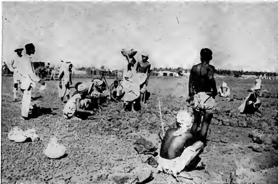
Women as well as men carry rock for the runway of a new airfield
